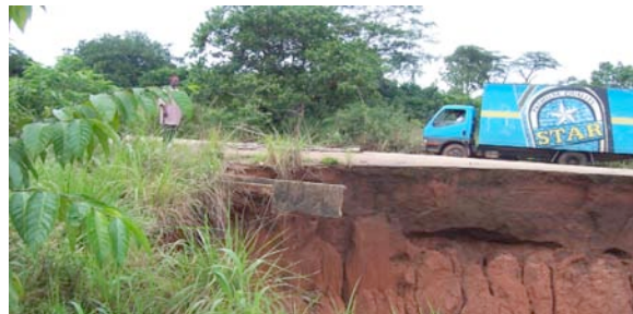
Figure 2. A Gully at Uturu-Kanu Road near Abia State University, Uturu.
